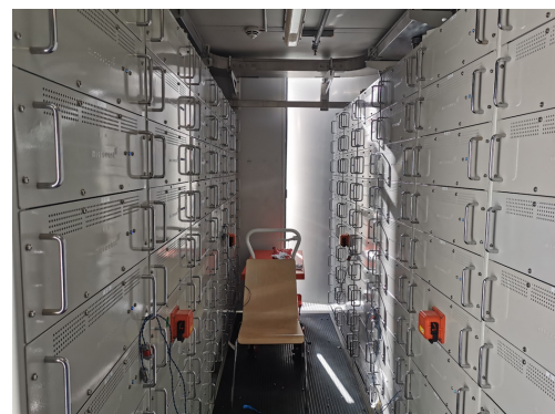
Fig. 1. Inside view of the LTO container
